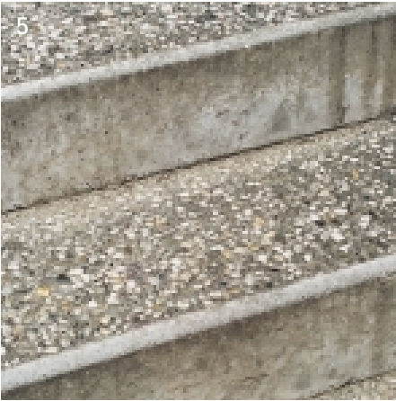
5. An attractive stair detail using fairface concrete risers with exposed aggregate treads.
