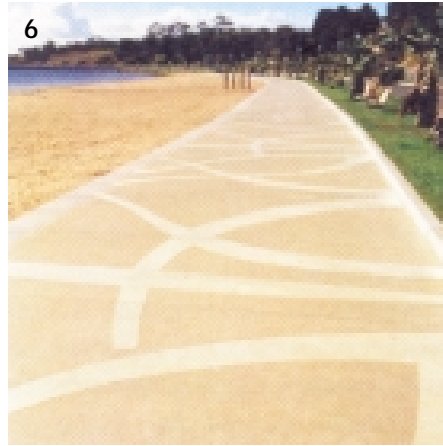
6. Pattern created using steel stencils laid out prior to abrasion blasting. Photo courtesy of C&CAA.
