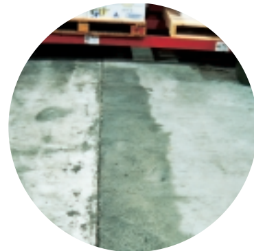
Hand trowelled section adjacent to the construction joint is considerably less durable than the rest of the slab. Bleed water/cement paste may have been mixed at edges.
