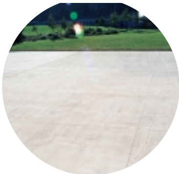
Early thermal shock crack in exterior concrete slab. Note the slab run adjacent to the saw cuts suggesting the crack was present before the saw cutting operation.
