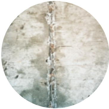
Joint failure. Pallet stackers with solid tyres are causing the epoxy nosing to pull away from the adjacent 25MPa concrete.
