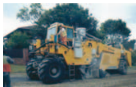
A Wirtgen stabiliser/reclaimer 2500k stabilising using the conventional spread and mix construction technique.
