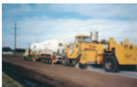
A Wirtgen 2500k construction on a deep lift pavement, with a lime binder. Note the binder tanker in front allowing the direct injection of binder into the ground without dust emissions.
