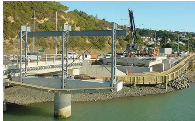
Super-T precast bridge beams are being used to construct the second Paremata Bridge (designed by Beca Carter Hollings and Ferner Ltd and built by Juno Civil Ltd for Transit New Zealand) on State Highway One near Wellington.
