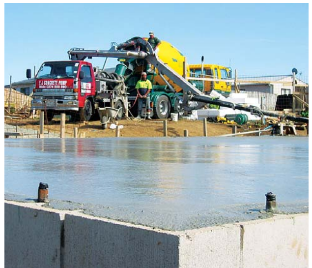
Pouring of floor slab (post-tensioned couplers shown extending out of the foundation).
