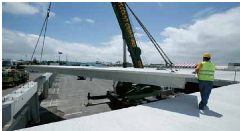
Above: The carpark's 17 metre long panels are eased into place at the AIAL carpark.
