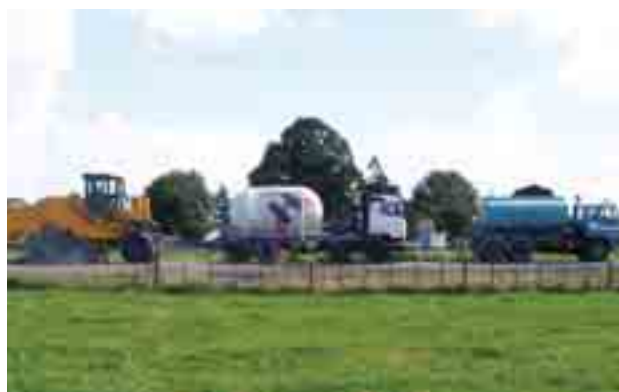
Fig. 2: The recycling train consisting of the WR 2500 SK pushing the powder tanker and the water tanker, which are all coupled together by push bars. The cement and water are transferred from the supply tankers to the recycler through flexible hoses.
