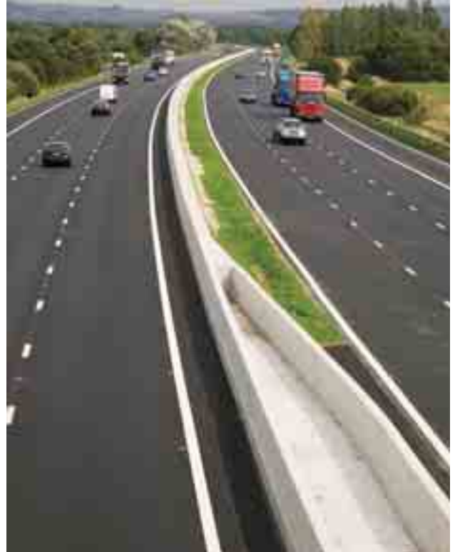
An example of an effective concrete step barrier in the UK. Image courtesy of Britpave.
