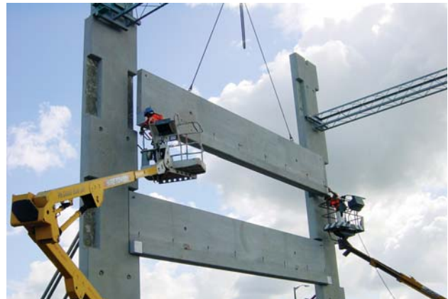
Assembly of Worldwide Parking Group Ltd's car parking building at Auckland Airport.
