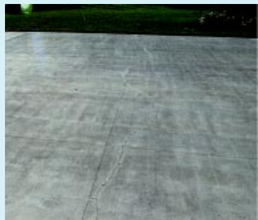
Figure 1 Note the wandering crack near the saw cut.
