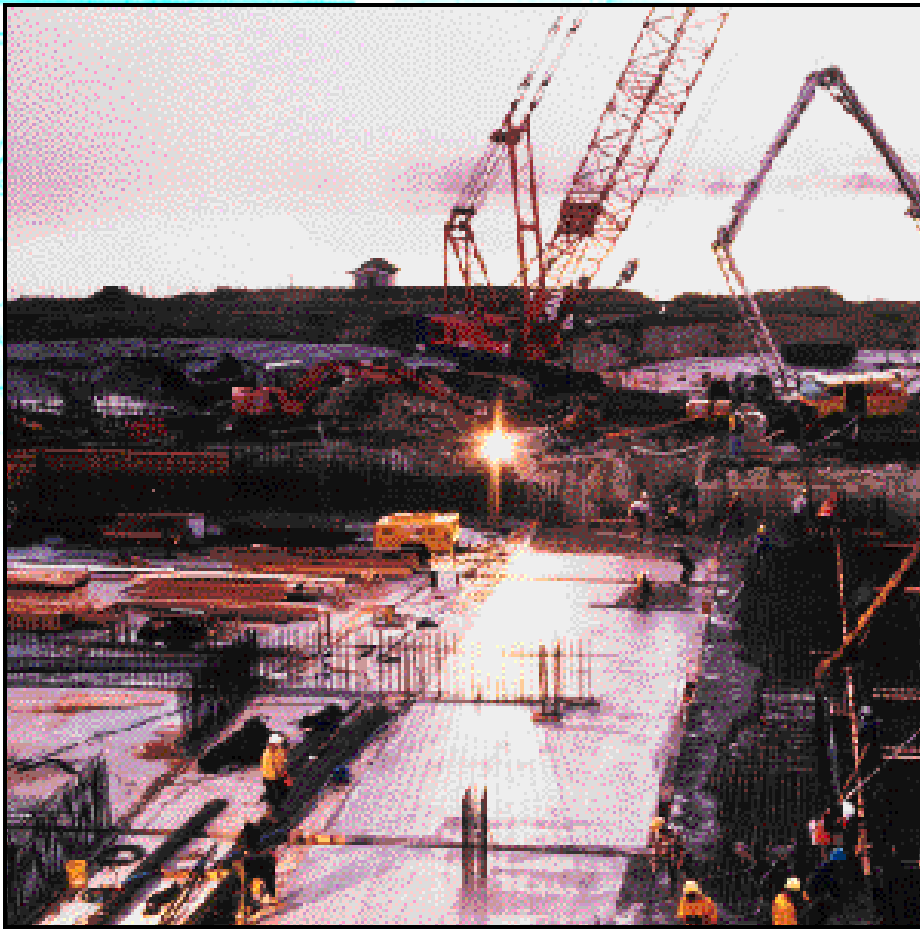
Above: The second of three main concrete pours at dawn for the floor of the MLE Tank.
