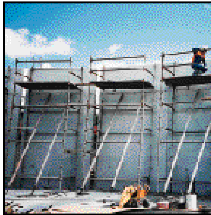
Inside view of the clarifier showing concrete mushroom, sloping floor, outside wall with precast concrete weir units attached, and clarifier outlet structure.
